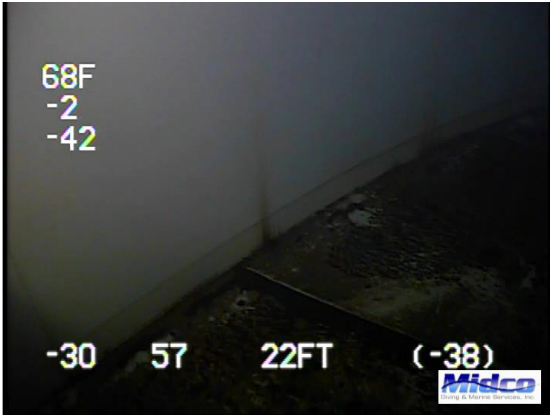
Floor to Wall Seam – Coating Failure with Corrosion Noted
