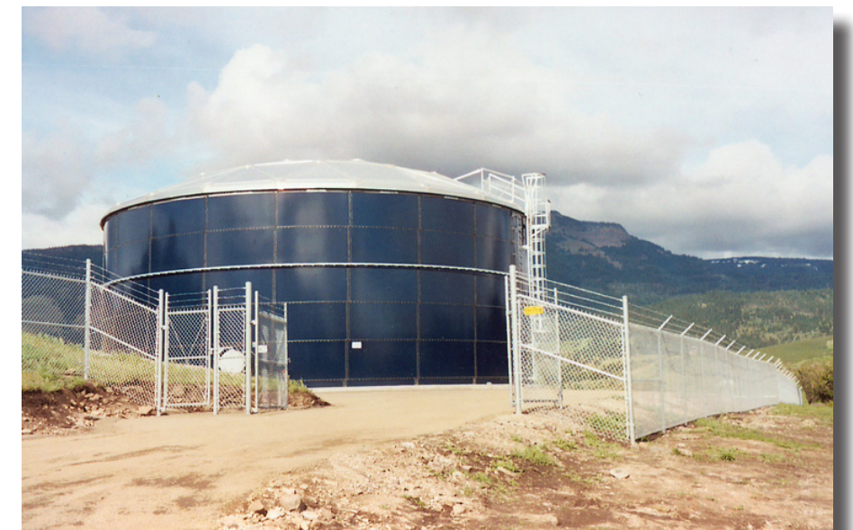
Ground Level Bolted Steel Reservoir - Cove, Oregon
