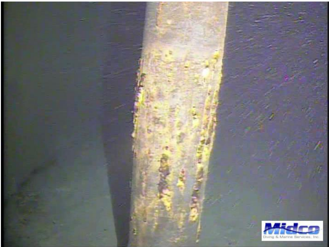
Overflow Plumbing – Corrosion Noted
