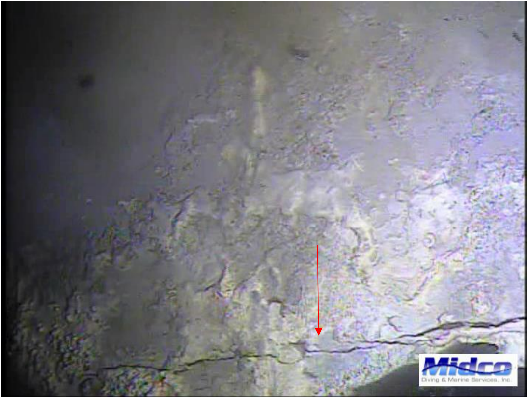
Areas with Repair Failures Noted
