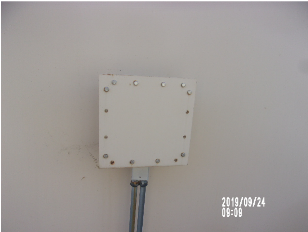
Exterior Telemetry – Hardware Corrosion Noted
