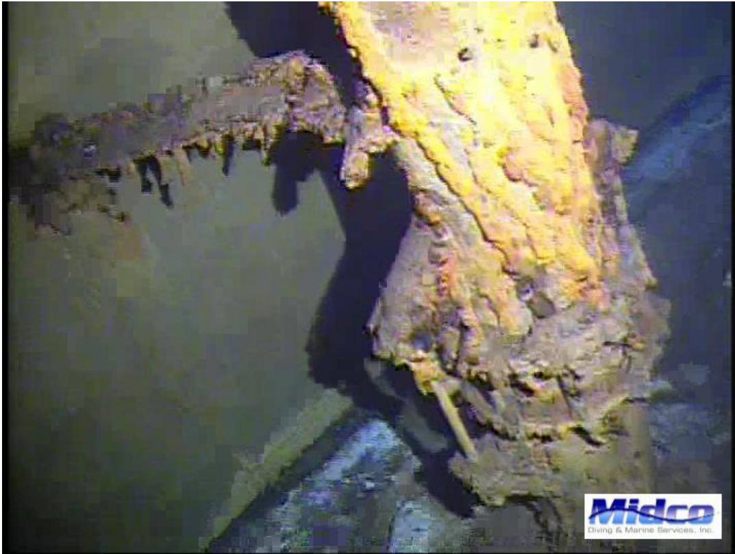
Overflow Plumbing – Coating Failure with Corrosion Noted
