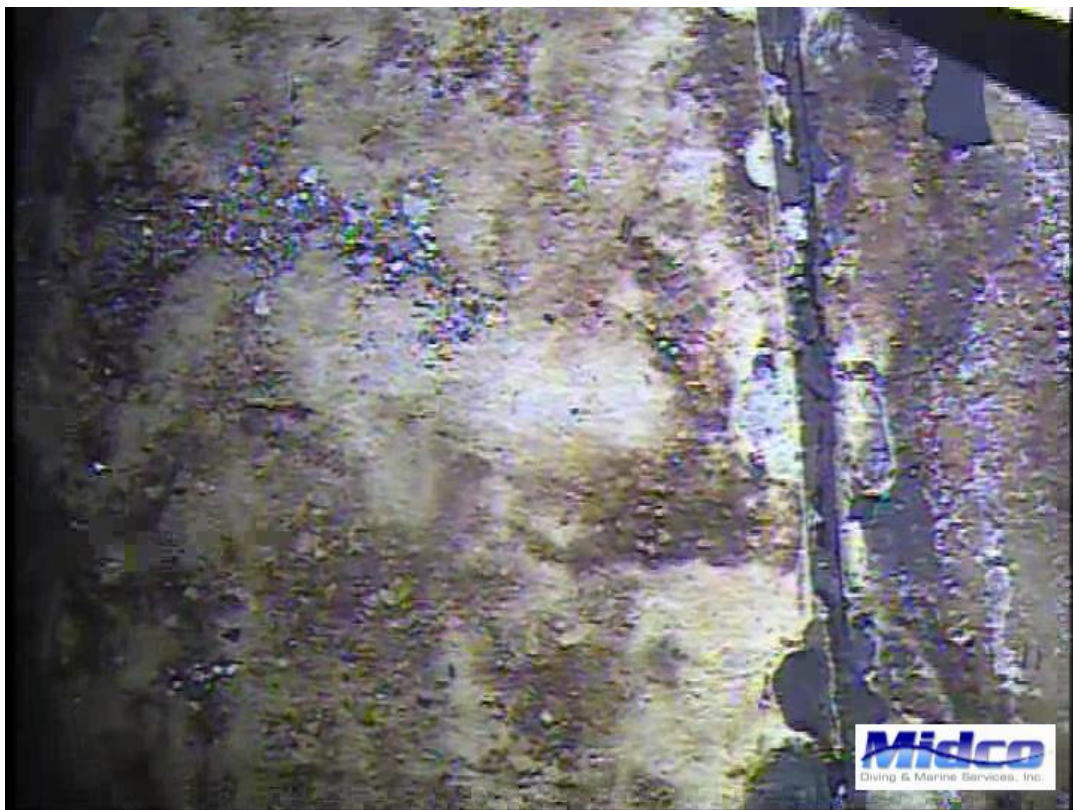
Seam Sealant Deterioration Noted
