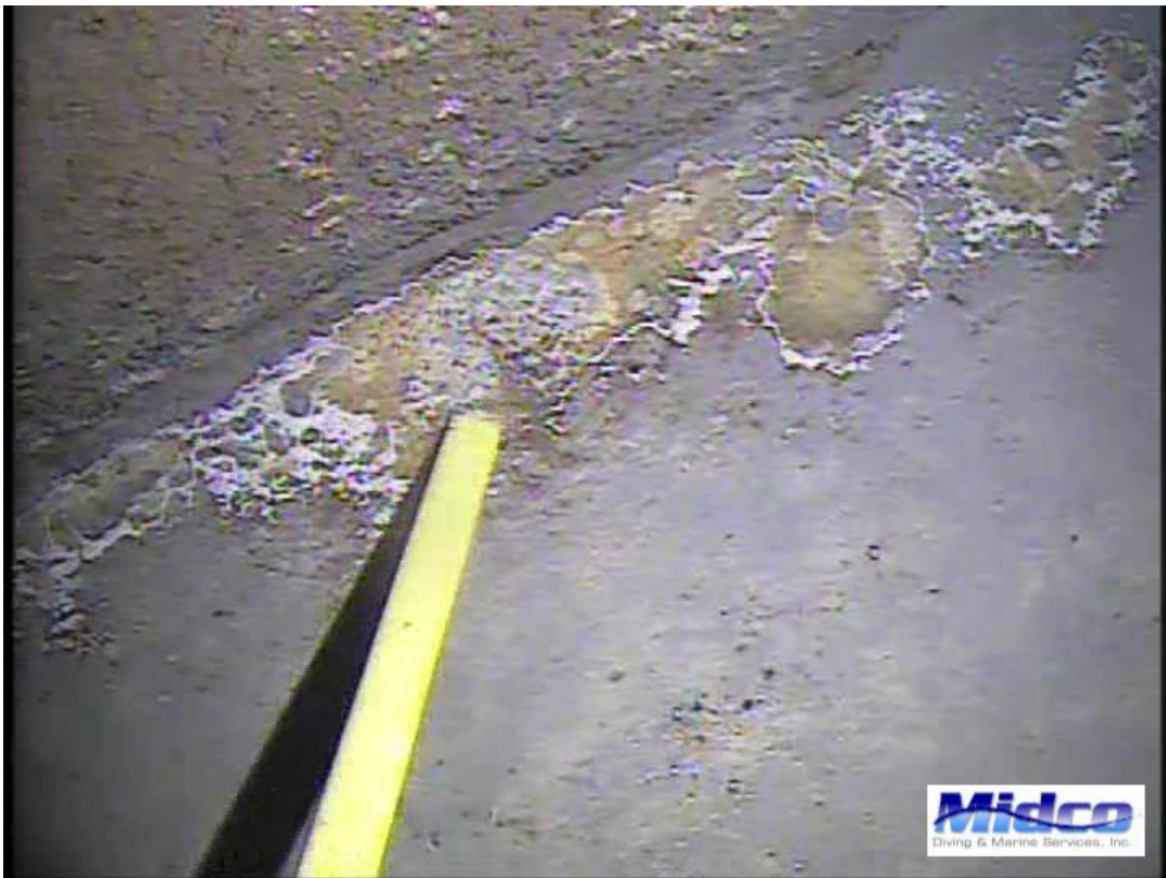
Floor to Wall Seam
