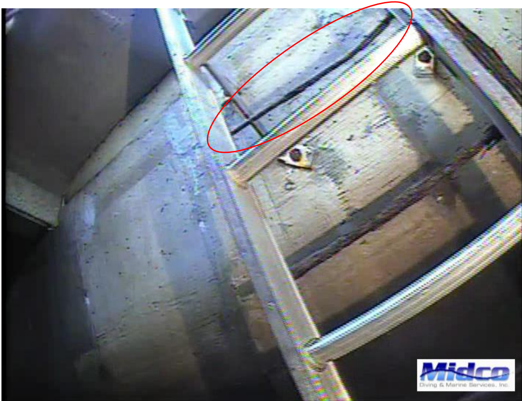
Ladder Rung Deterioration Noted
