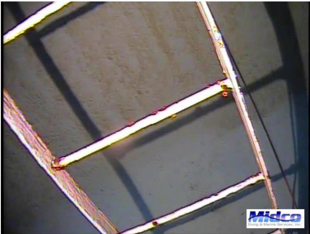
Interior Ladder – Coating Failure with Corrosion Noted
