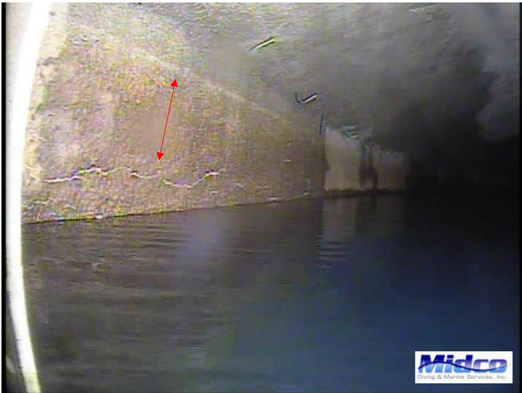
Wall to Roof Seam – Settling Cracks Noted
