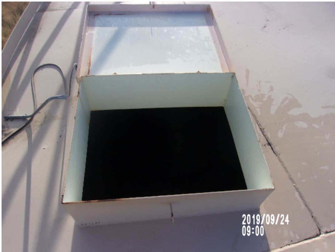
Access Hatch – No Weather Stripping Noted
