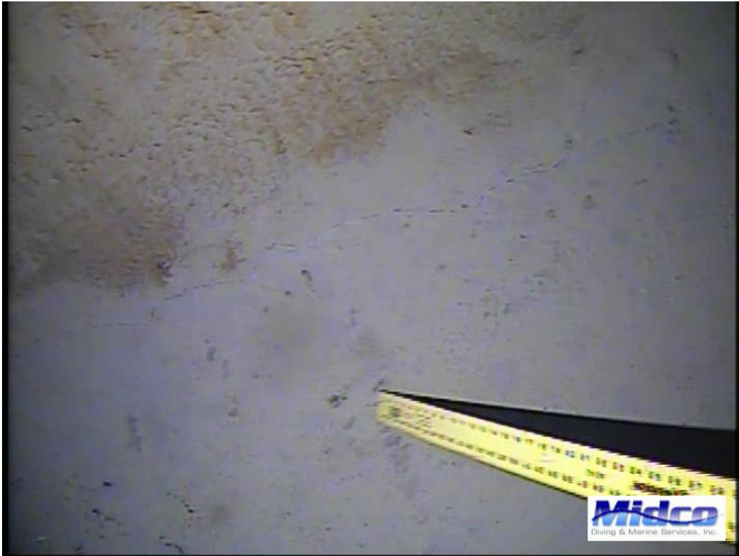
Floor to Wall Seam
