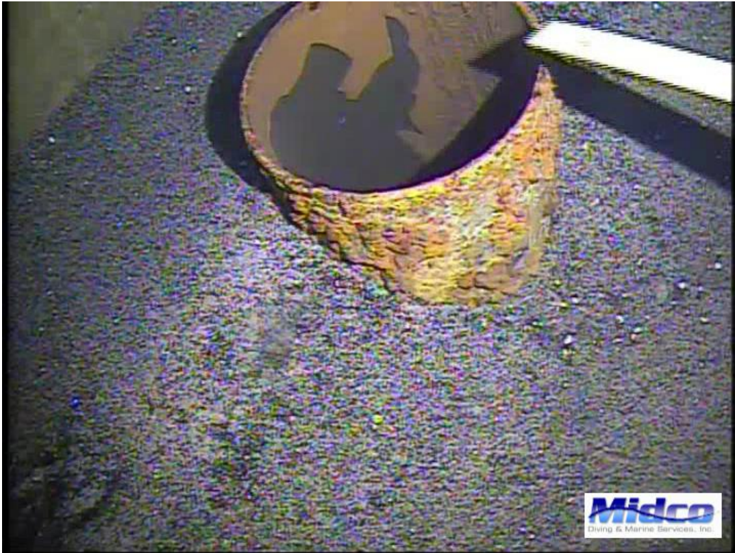
Inlet Plumbing – Coating Failure with Corrosion Noted
