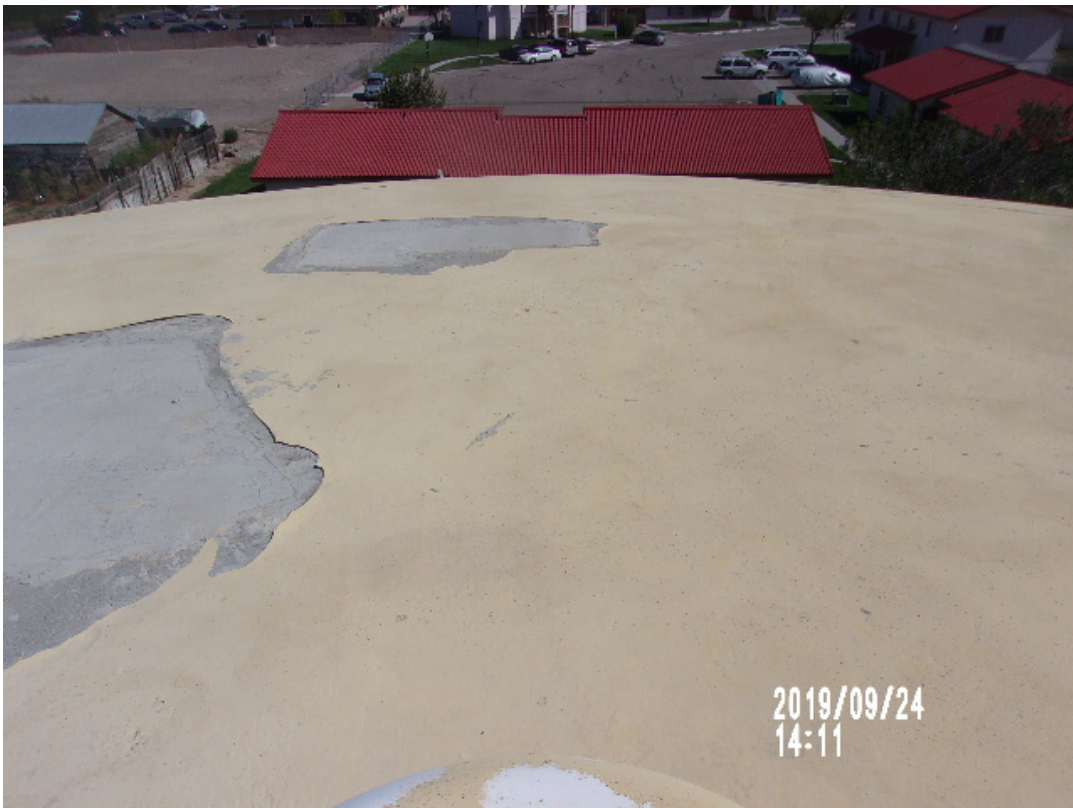
Reservoir Roof – Coating Failure Noted
