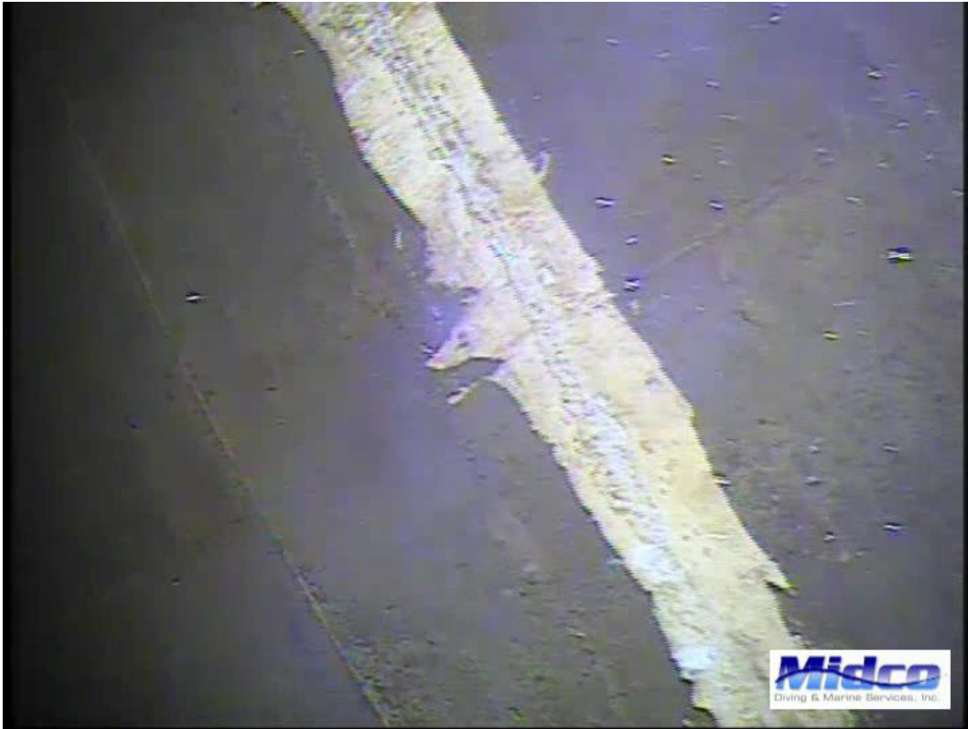
Previous Repairs Noted
