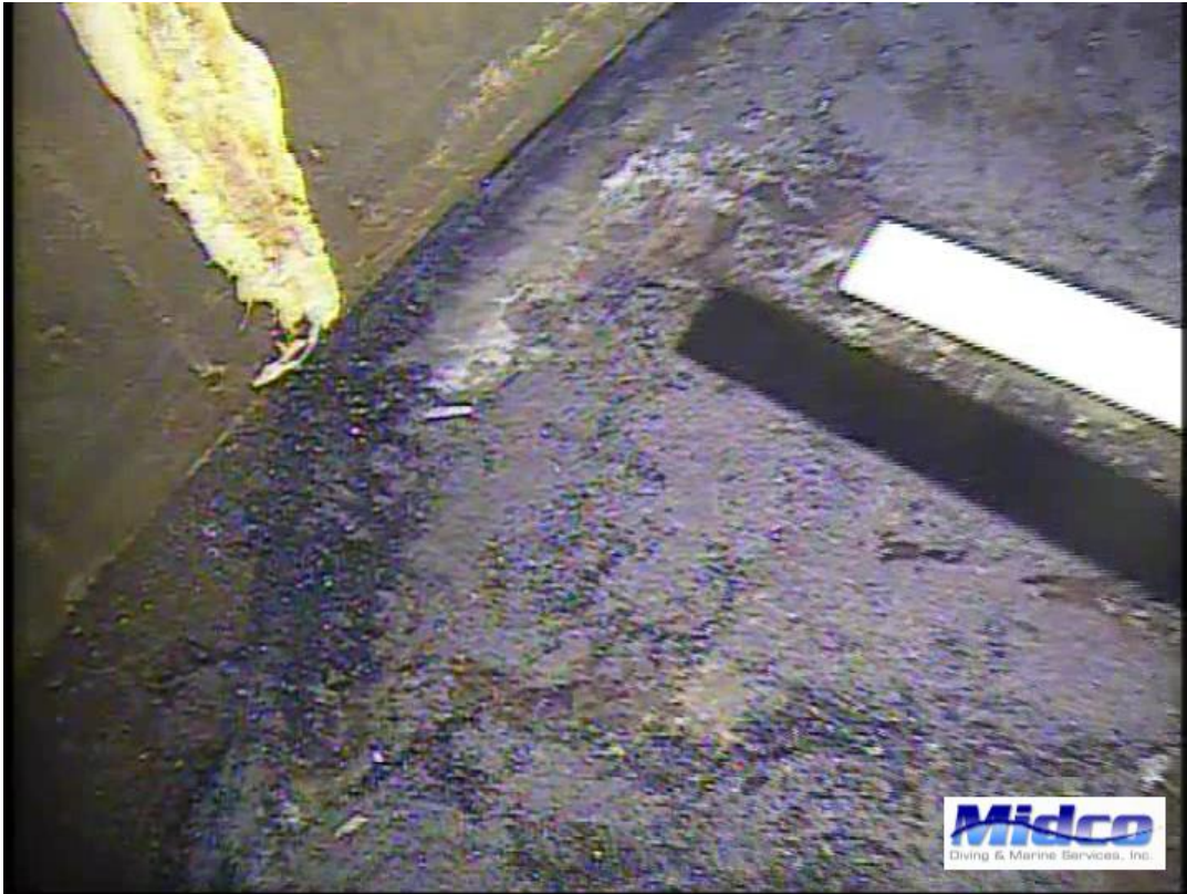
Floor to Wall Seam
