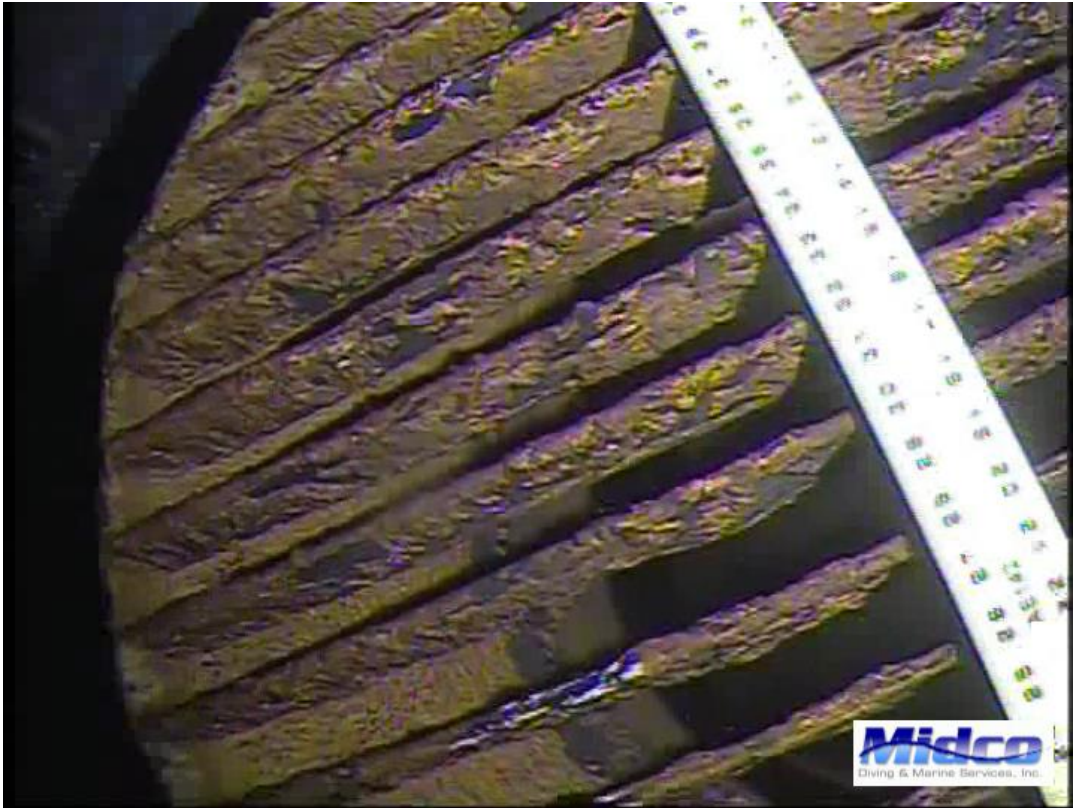
Outlet Plumbing – Coating Failure with Corrosion Noted
