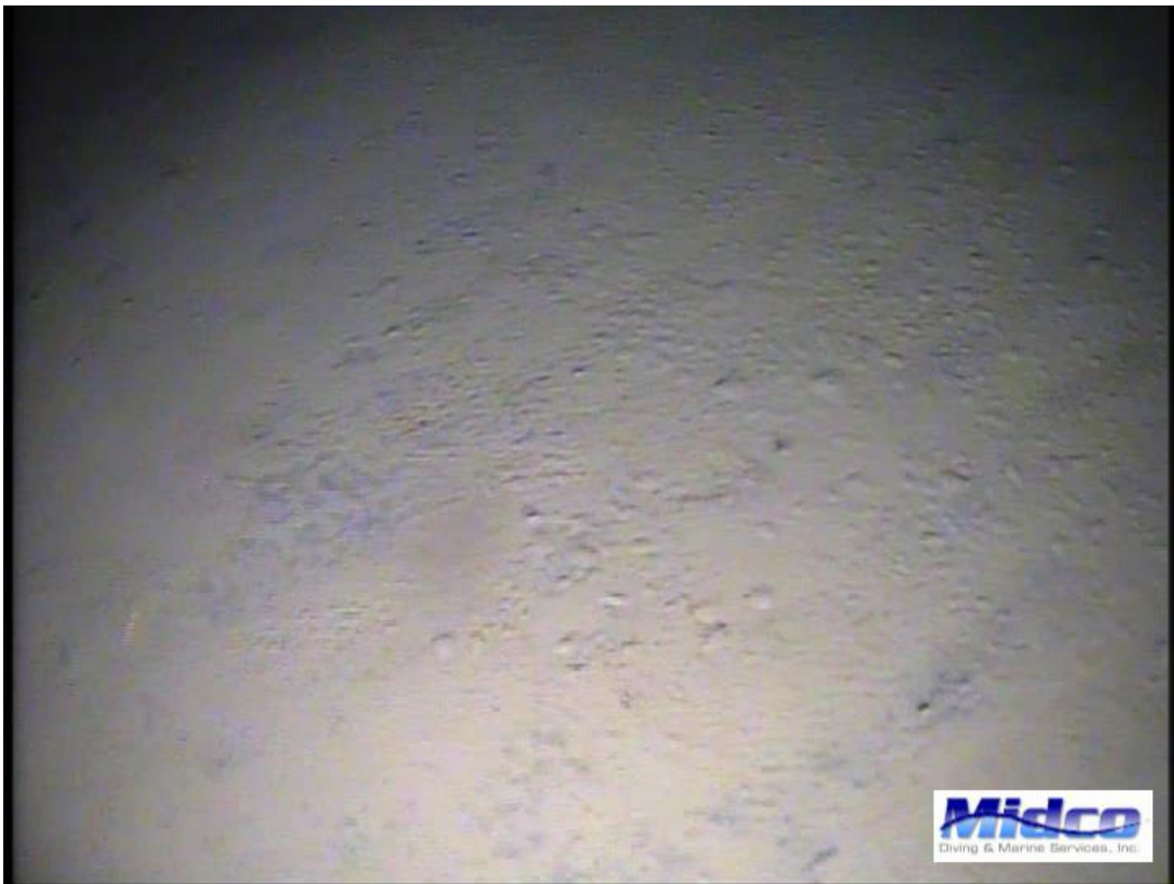
Typical Floor – Coating Failure Noted
