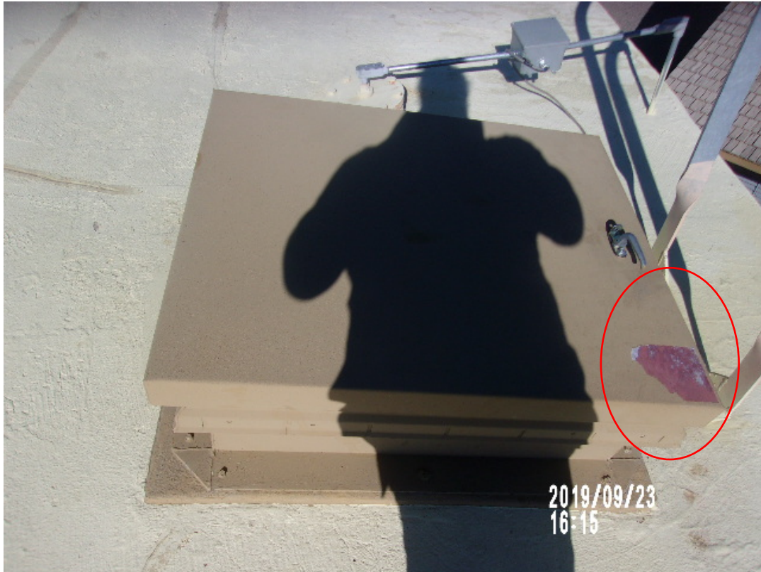
Access Hatch – Coating Failure Noted
