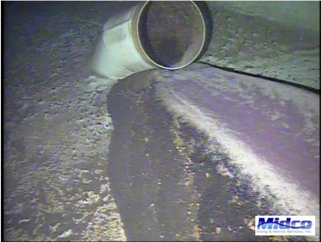
Up to 20" of Sediment Noted Near Inlet Plumbing – Possible Filter Rupture
