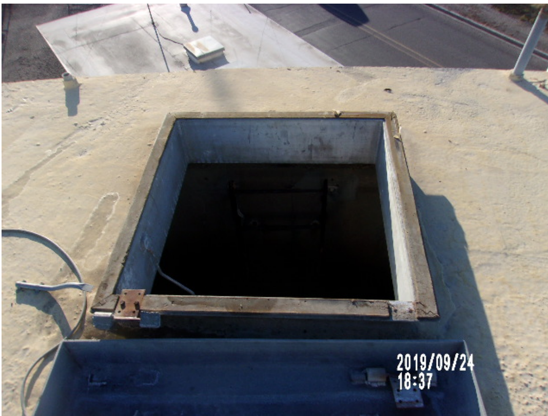
Access Hatch – Hinge Deterioration Noted
