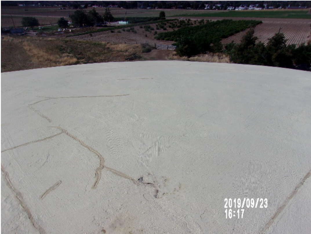
Reservoir Roof – Settling Cracks Noted
