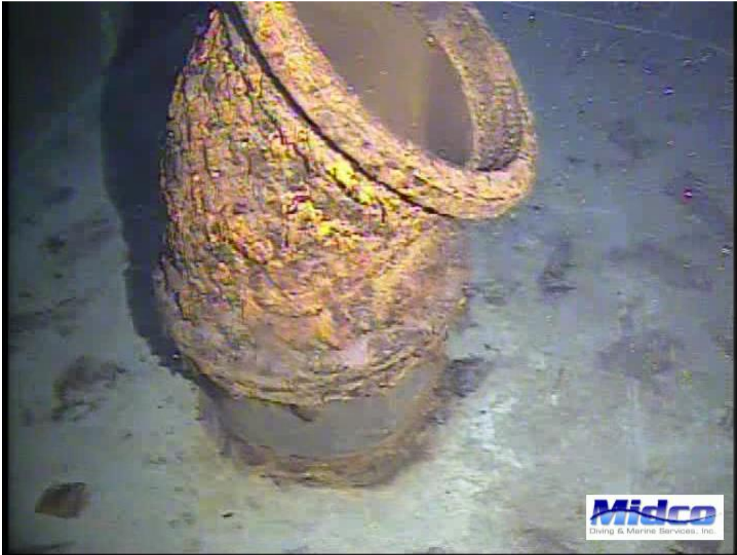
Inlet Plumbing – Corrosion Noted
