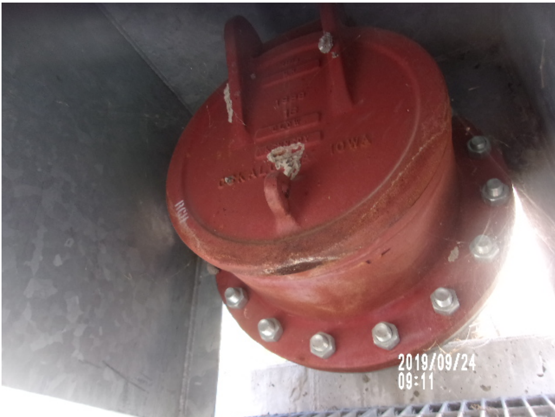
Overflow Plumbing Flapper Valve
