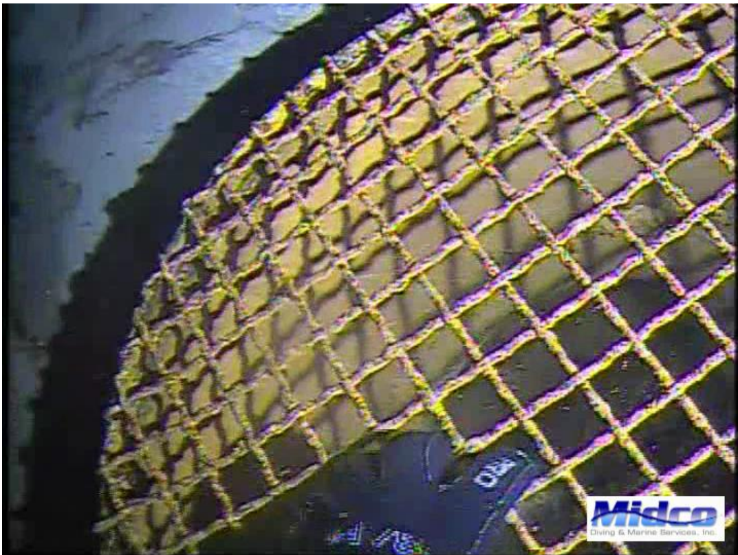
Outlet Plumbing – Corrosion Noted
