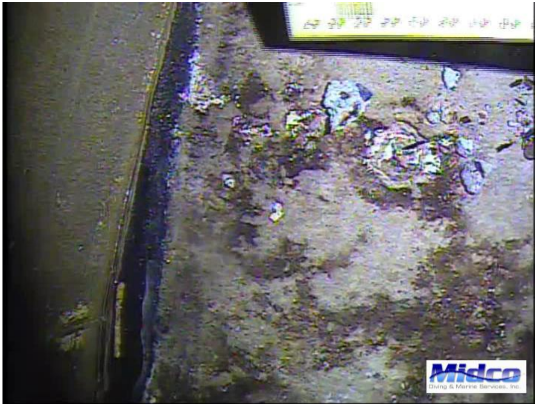
Areas of Spalling Noted
