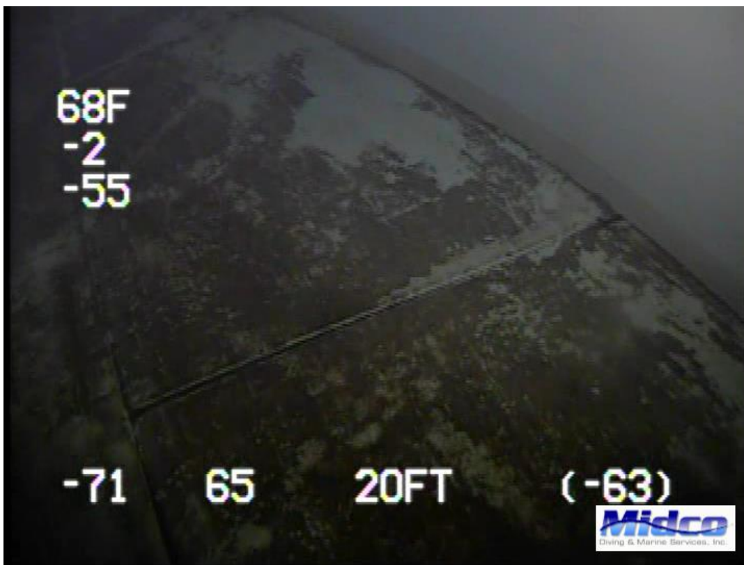
Floor to Wall Seam
