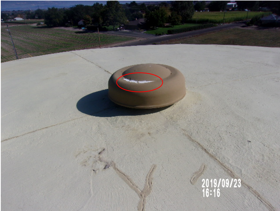
Roof Vent – Coating Failure Noted
