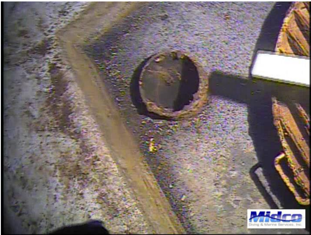
Drain Plumbing – Coating Failure with Corrosion Noted
