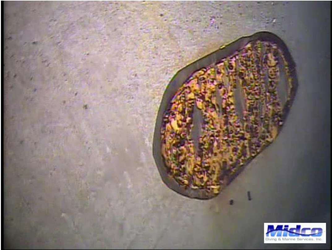
Interior Plumbing – Corrosion Noted
