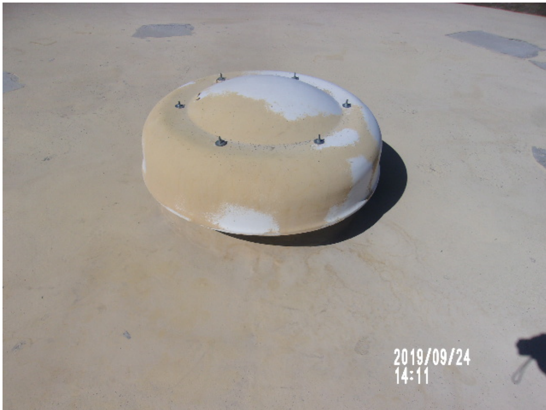
Roof Vent – Coating Failure Noted
