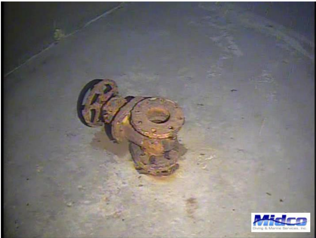
Interior Plumbing – Corrosion Noted
