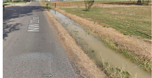
Open Ditch Along Dorian Dr. (Source: Google Streetview)
